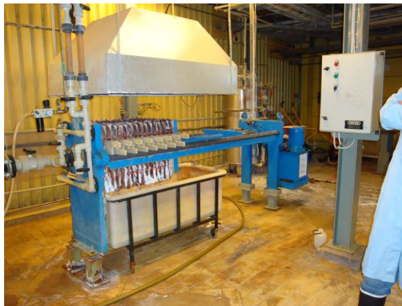
Figure 2-10 Filter Press for Leaching Residues
