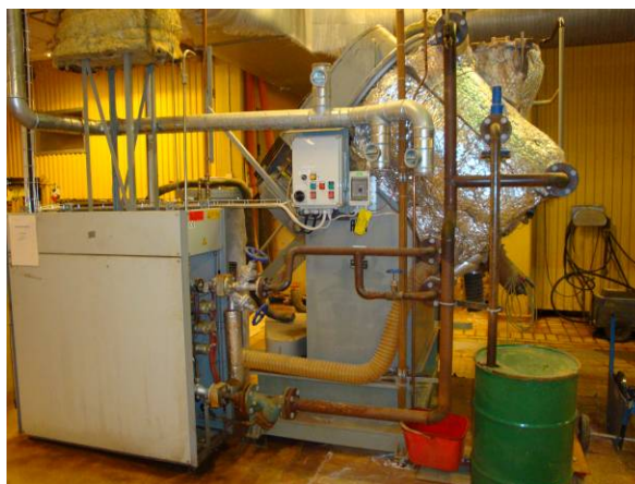
Figure 2-16 Drying Equipment for Leaching Residues
