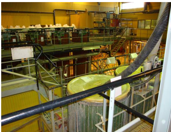
Figure 2-7 RMA Leaching Hall Showing Storage Tanks in Background
