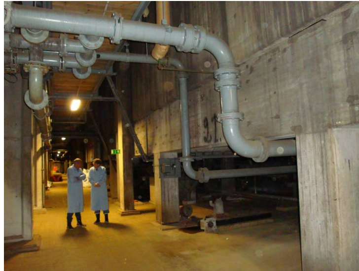
Figure 2-5 Basement of Large Leaching Hall Showing Liquor Management Pipework
