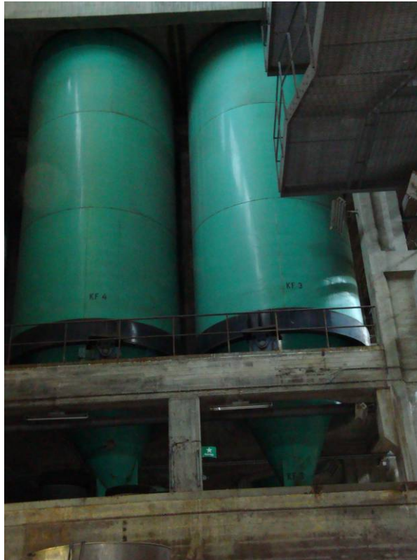
Figure 2-23 Dust Collecting Tanks in Old Sorting Facility
