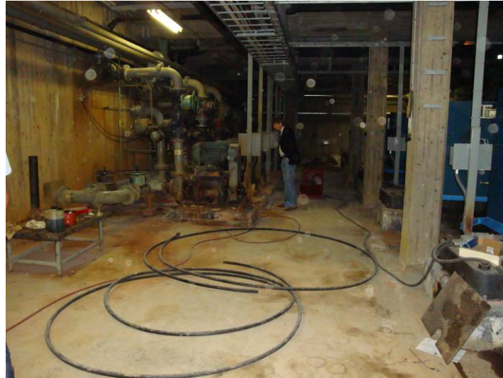
Figure 2-25 One of the Basement Rooms in Control Building
