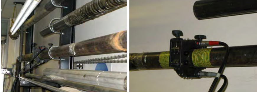
Figure 4.2: Transducer ring installed on the pipe mockup used in the demo-test (left). Transducer half-rings attached in mechanical contact with the tube wall (right).
