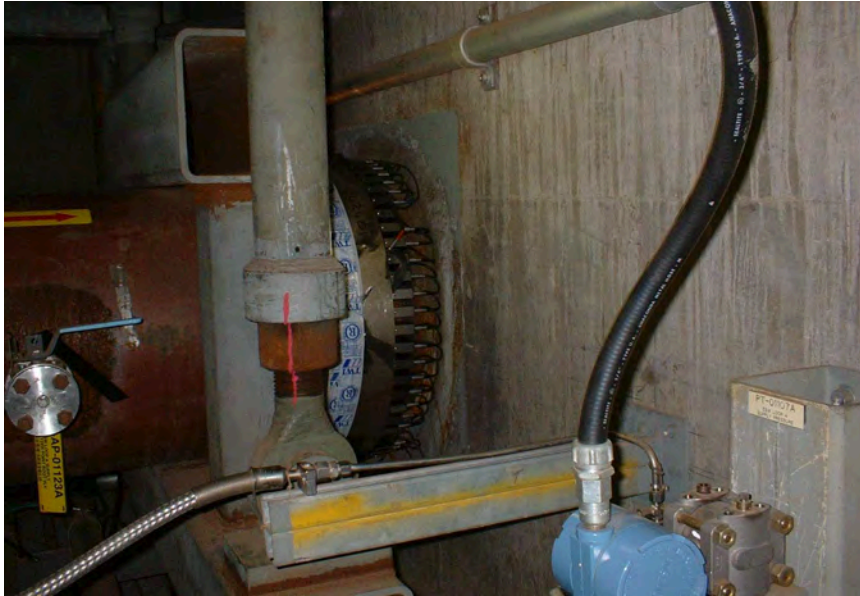
Figure 3.20: Teletest installation on a 24" emergency cooling water pipe at a nuclear plant.
