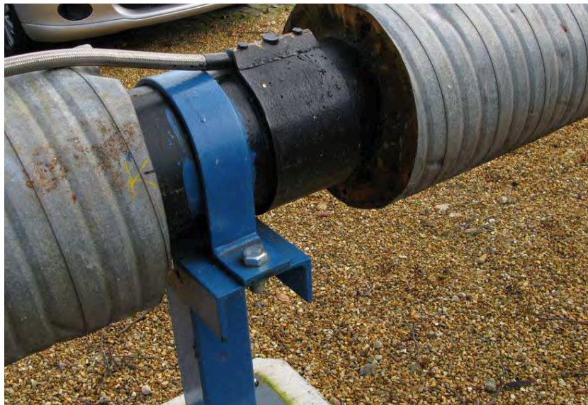
Figure 3.19: Example of an encapsulated transducer ring developed by Plant Integrity Ltd.
