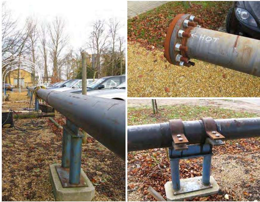
Figure 4.5: TL01 pipeline tested in the TWI demo-test (left). Flange on eastern end of line (upper right) and one of the supports (lower right).
