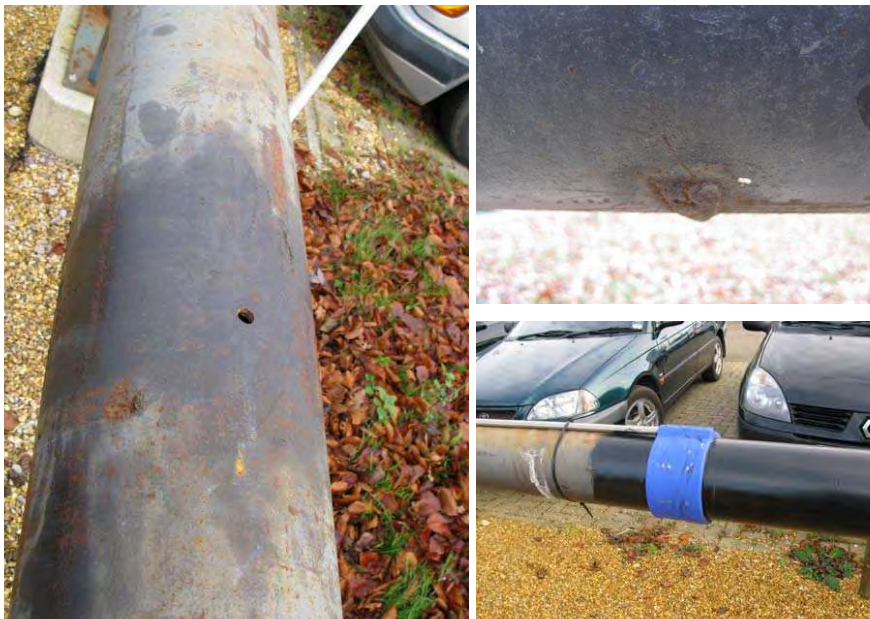
Figure 4.7: Artificial defects in TL01 pipeline tested in the TWI demo-test. Drilled hole in the upper part of tube (left). Welded plate on the lower part of tube (upper right) and a permanent transducer collar. (lower right).
