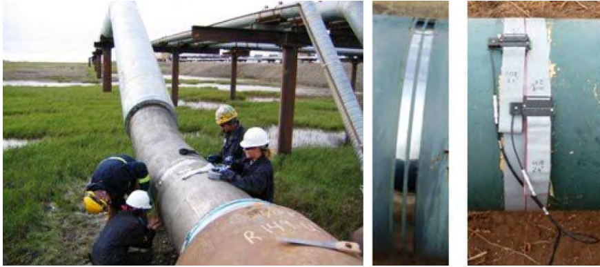
Figure 3.21: Installation of MsS on a pipeline (left). Magnetostrictive bands (middle). Encircling coil formed of a ribbon cable (right).
