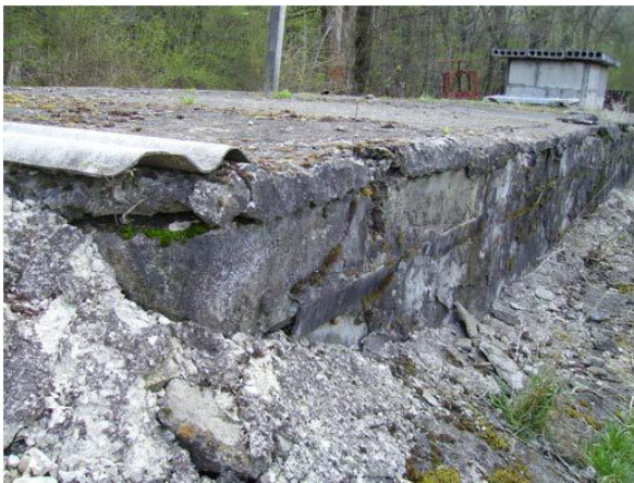
Fig. 7 Condition of the facility (Site Report, p.88).
